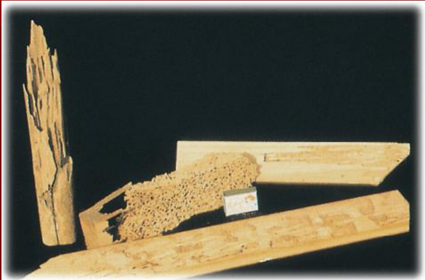
Severe subterranean termite attack to building timbers.
